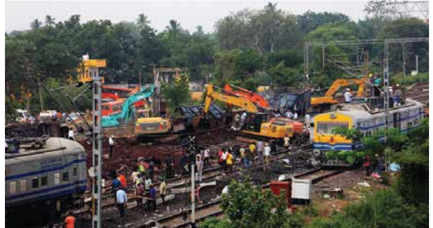
Fast-paced work: Workers busy restoring the track at the accident spot at the Bahanaga railway station in Balasore district of Odisha on Sunday. BISWARANJAN ROUT
